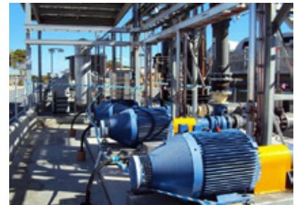
DAFT area recirculation pumps
